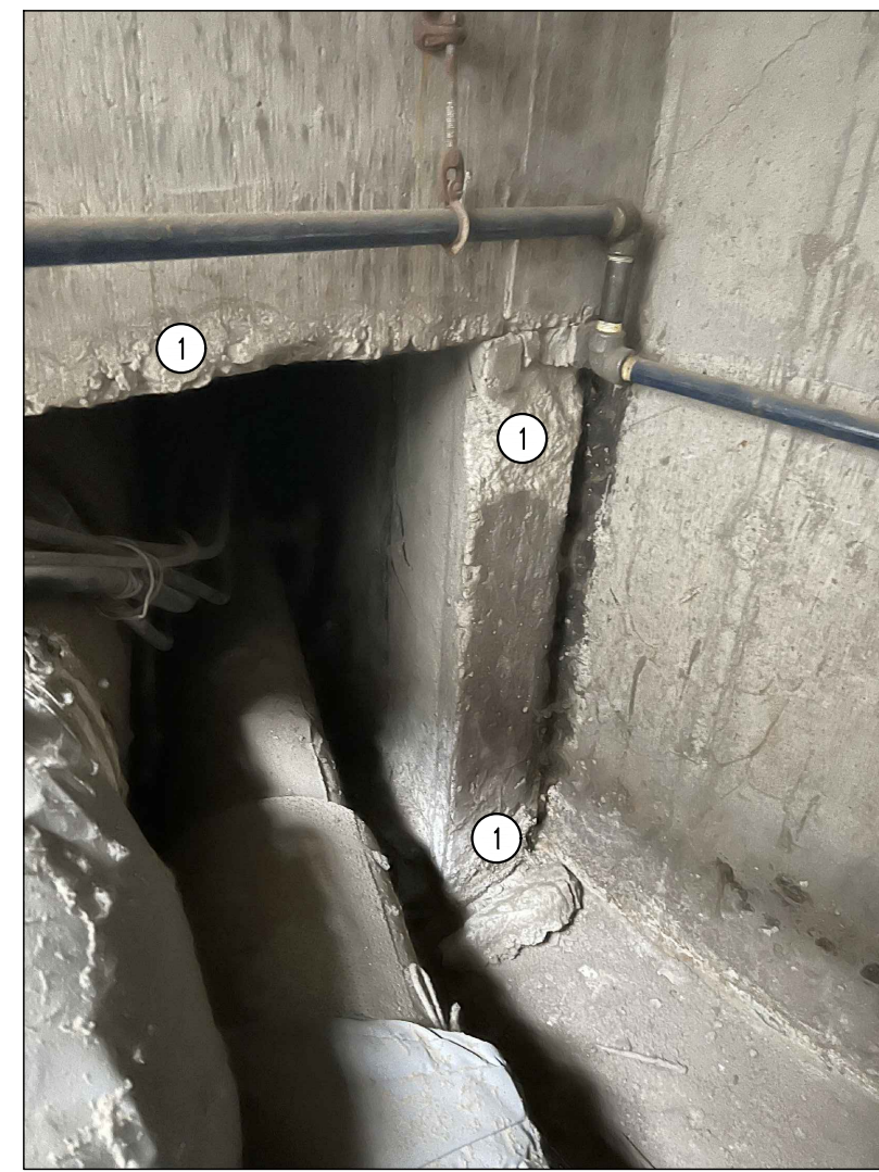
1 SPALLED CONCRETE, SEE REPAIR NOTE 2.
