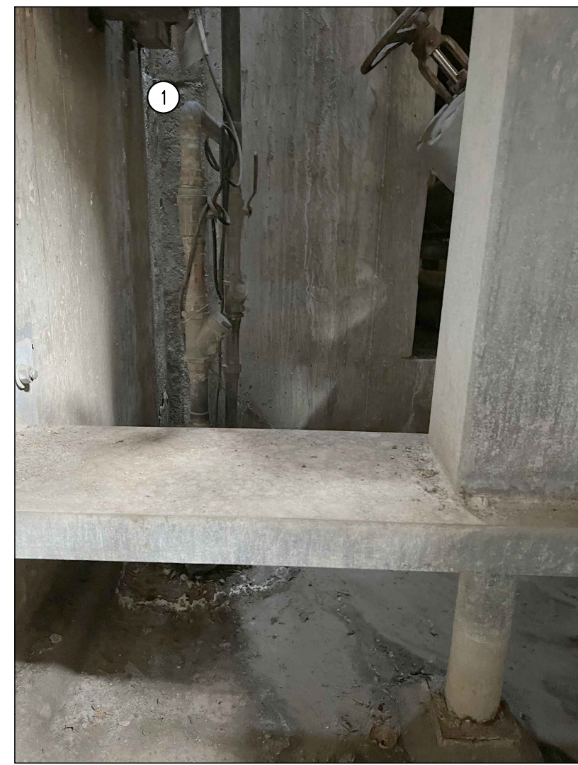
1 CONCRETE CRACKING, SEE REPAIR NOTE 1.
