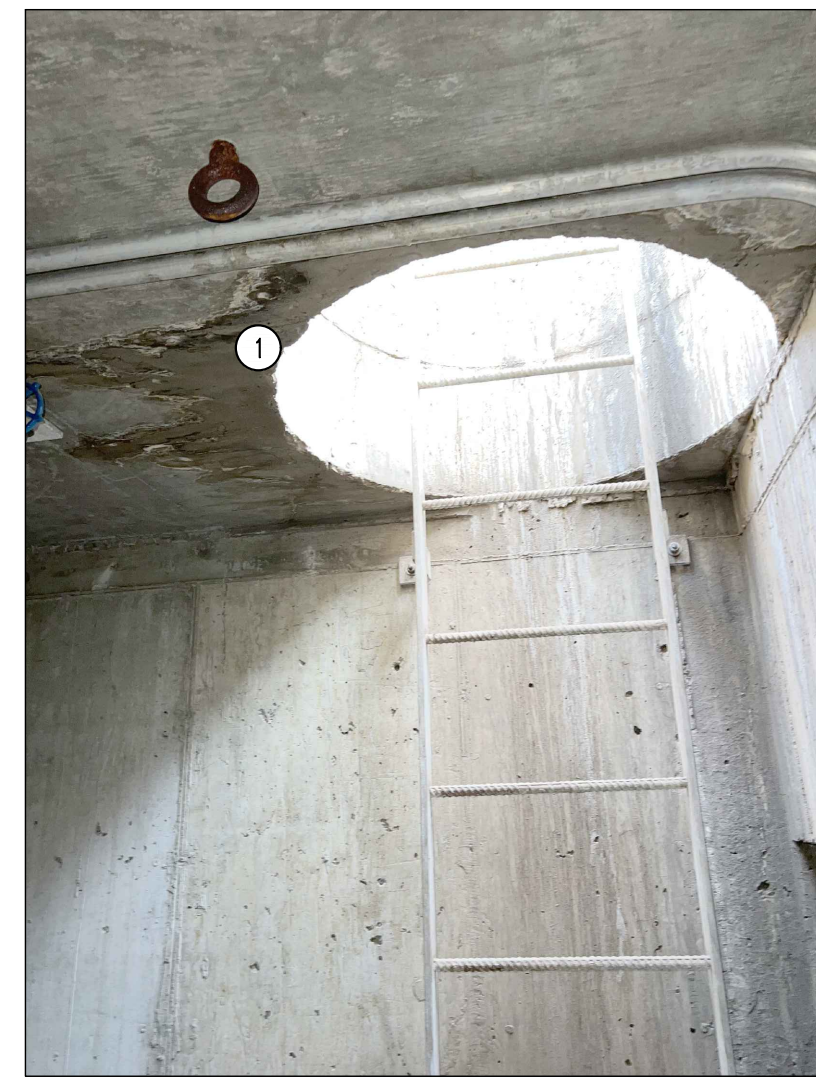
1 SPALLED CONCRETE, SEE REPAIR NOTE 3.
