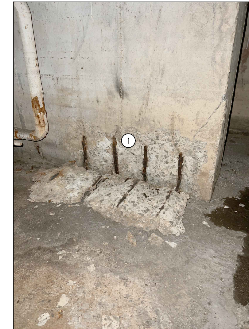
1 REBAR ANCHORAGE EXPOSED, SEE REPAIR NOTE 3.
