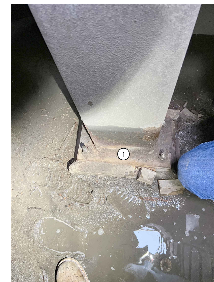
1 DAMAGED BASE PLATE, SEE REPAIR NOTE 1.
