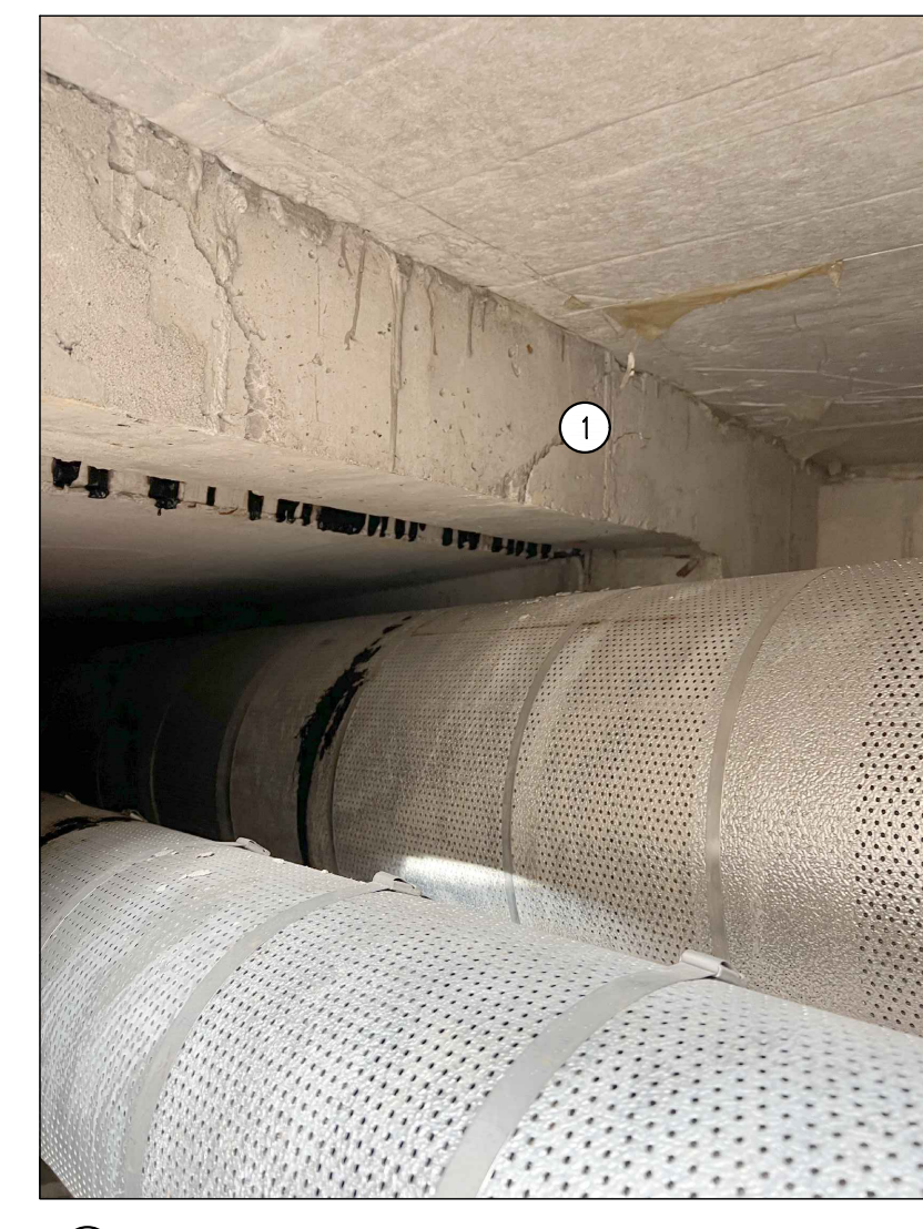
1 SPALLED CONCRETE, SEE REPAIR NOTE 4.
