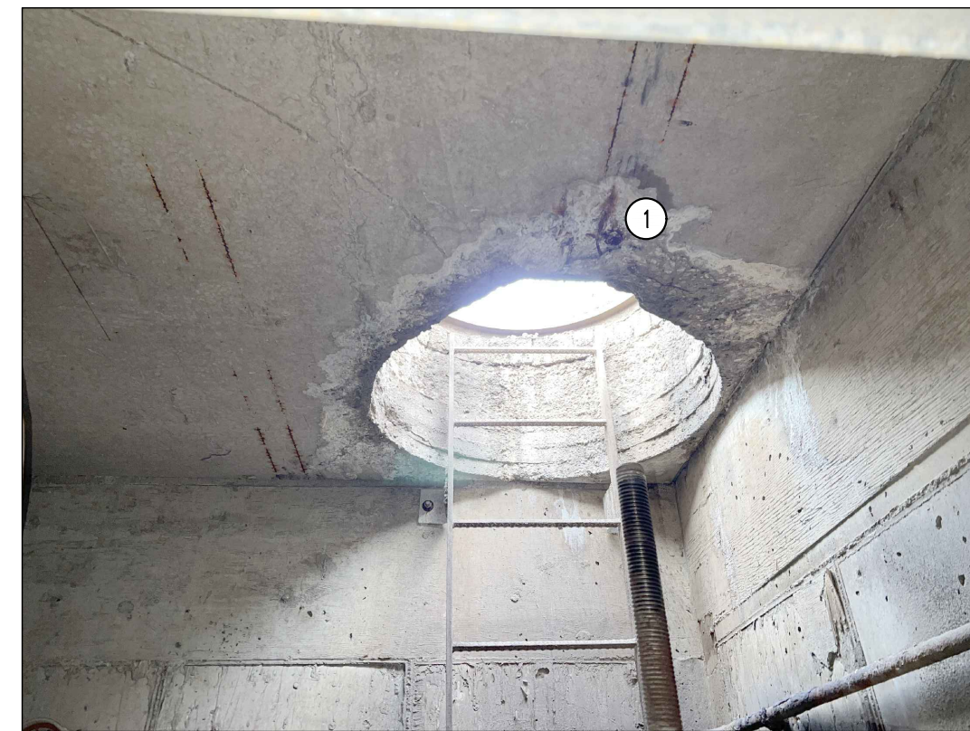
1 SPALLED CONCRETE, SEE REPAIR NOTE 1.
