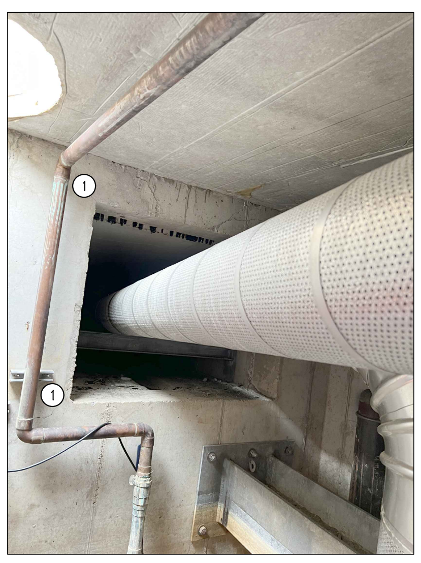
1 SPALLED CONCRETE, SEE REPAIR NOTE 3.
