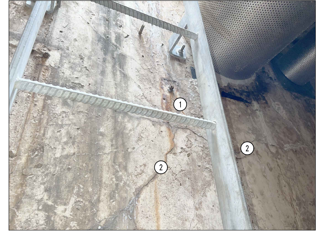
① SPALLED CONCRETE, SEE REPAIR NOTE 1. ② CONCRETE CRACKING, SEE CRACK REPAIR DETAIL ON SHEET S200.
