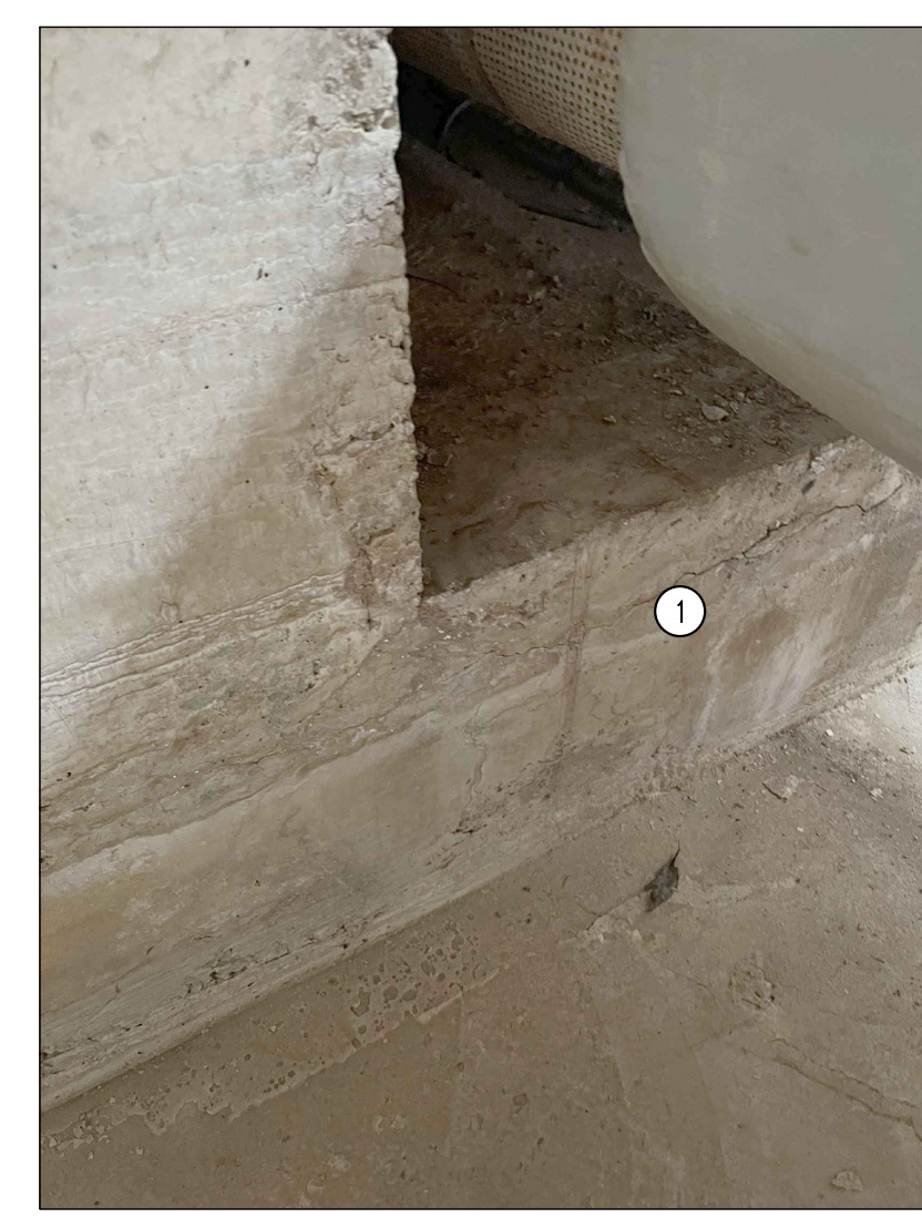
1 DEAD SPOT UNDER CHASE, SEE REPAIR NOTE 1.
