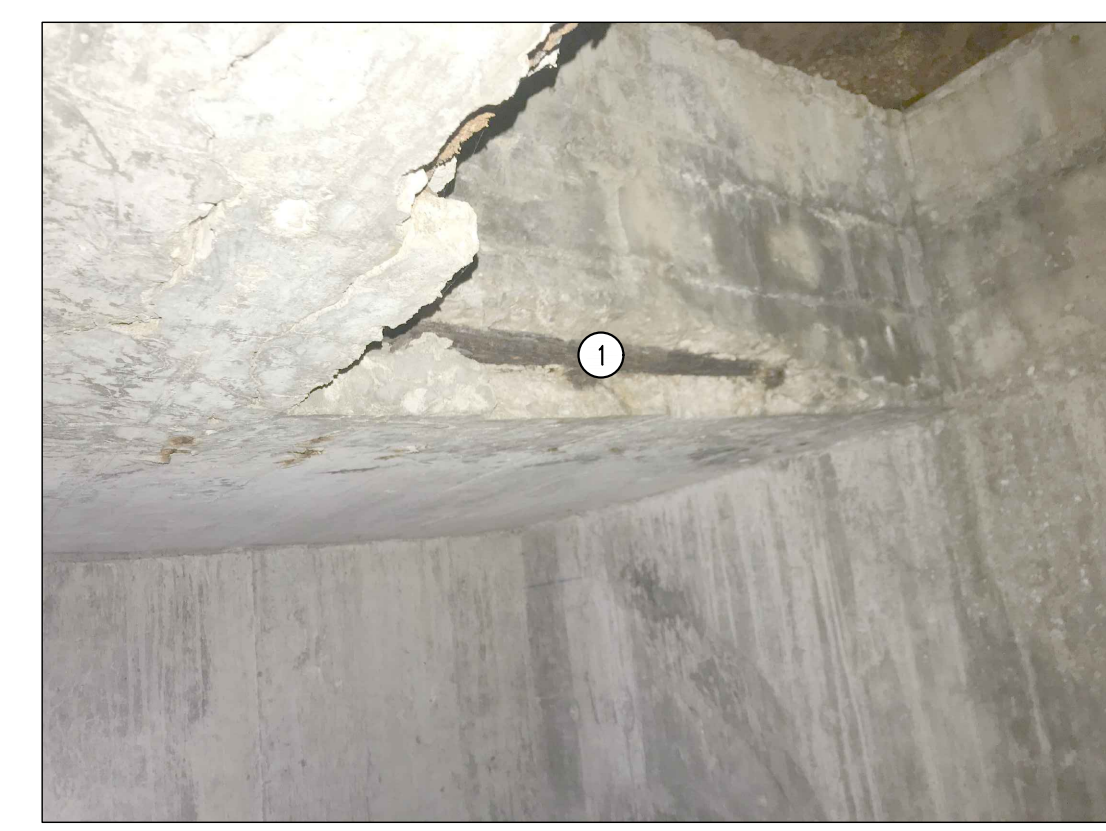
1 EXPOSED REBAR, SEE REPAIR NOTE 2.
