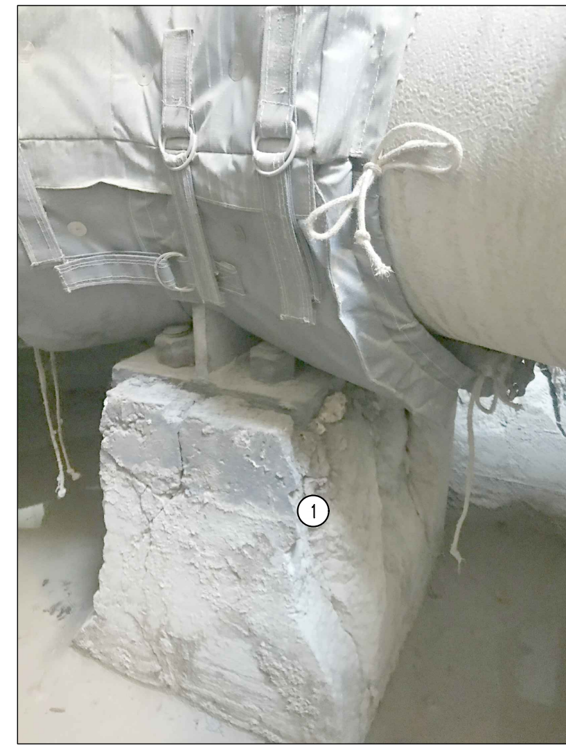
1 SPALLED CONCRETE, SEE REPAIR NOTE 1.
