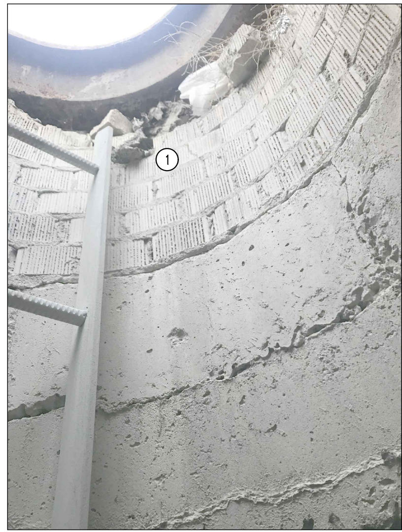
1 DAMAGED BRICK RISER, SEE REPAIR NOTE 3.
