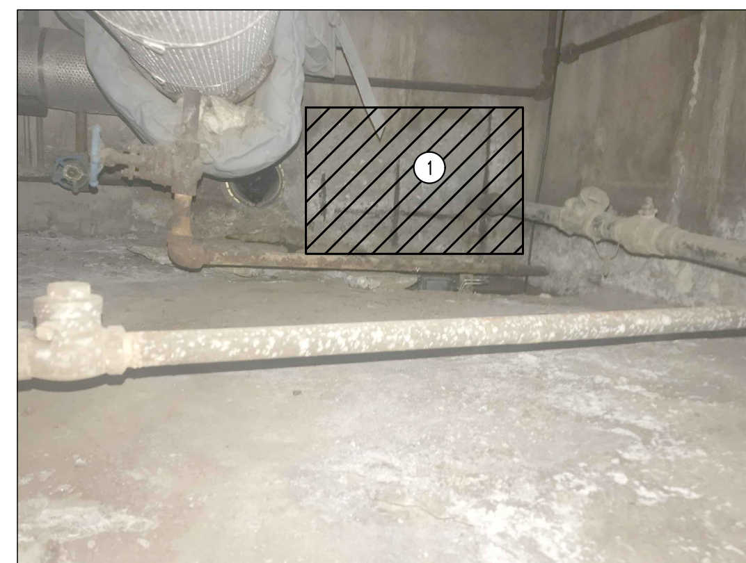
1 SPALLED CONCRETE, SEE REPAIR NOTE 6.
