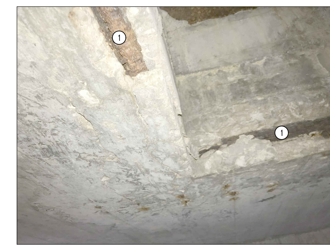
1 EXPOSED REBAR, SEE REPAIR NOTE 2.
