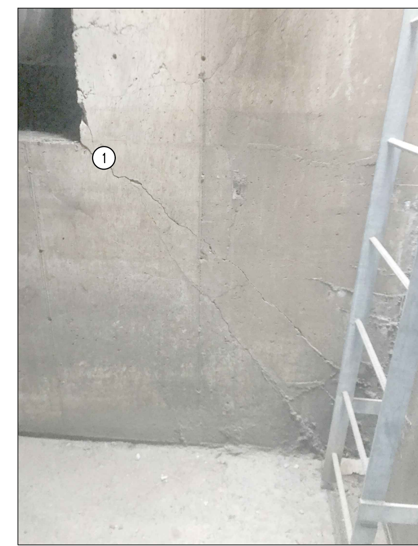
① SPALLED CONCRETE, SEE REPAIR NOTE 2.
