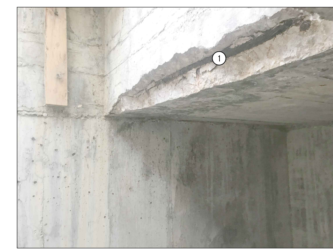
1 EXPOSED REBAR, SEE REPAIR NOTE 2.
