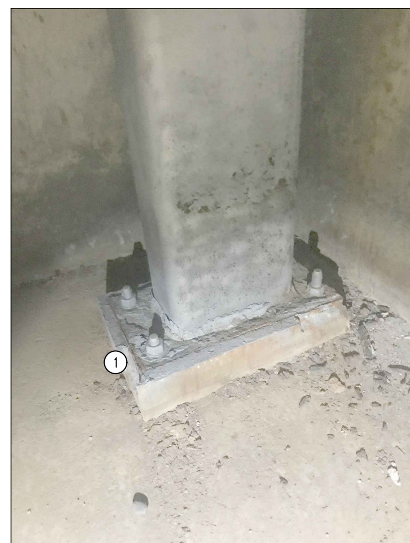
1 DAMAGED BASE PLATE, SEE REPAIR NOTE 2.
