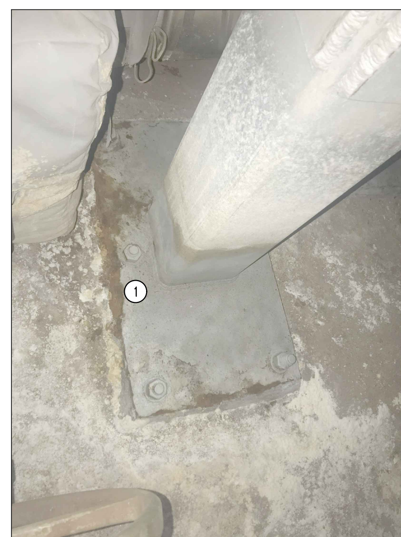
1 DAMAGED BASE PLATE, SEE REPAIR NOTE 2.
