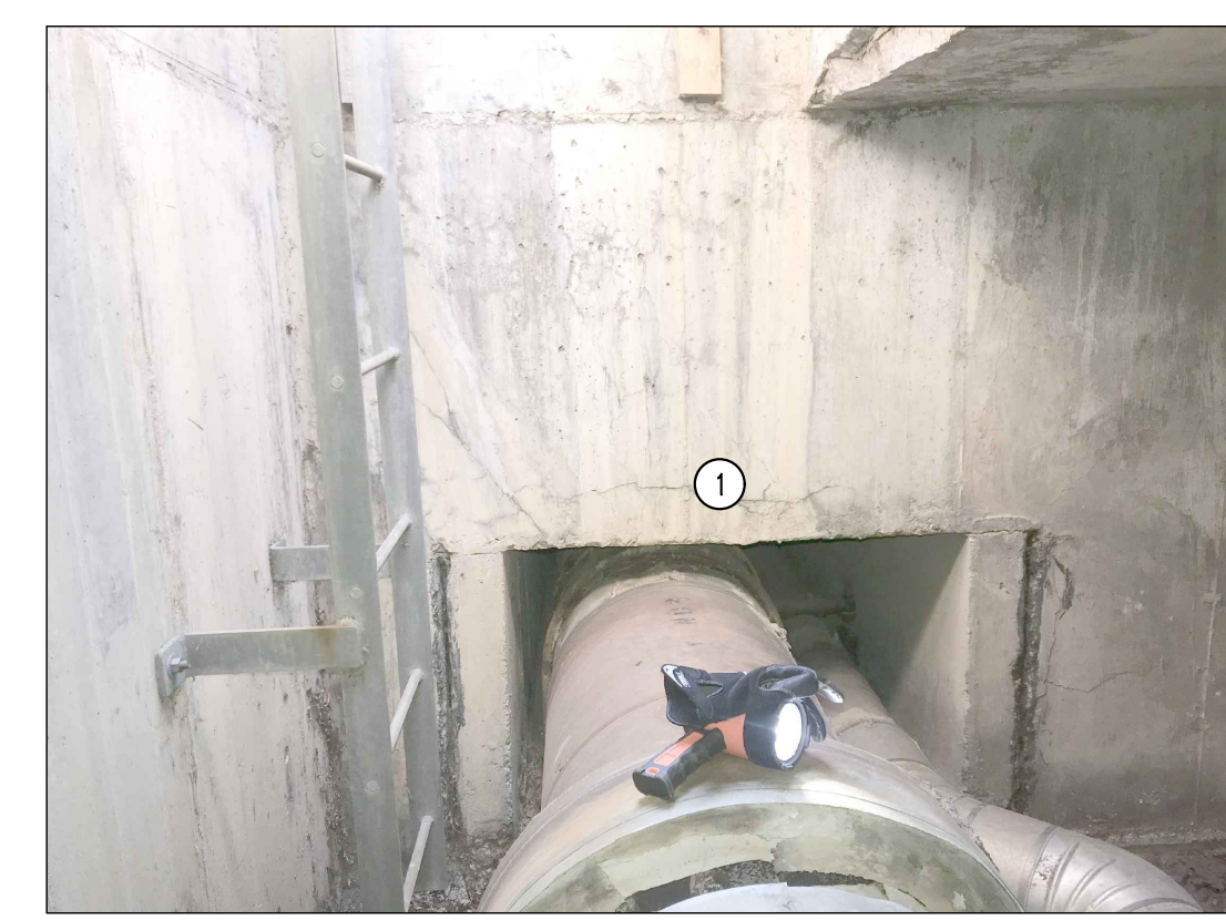
1 SPALLED CONCRETE, SEE REPAIR NOTE 4.
