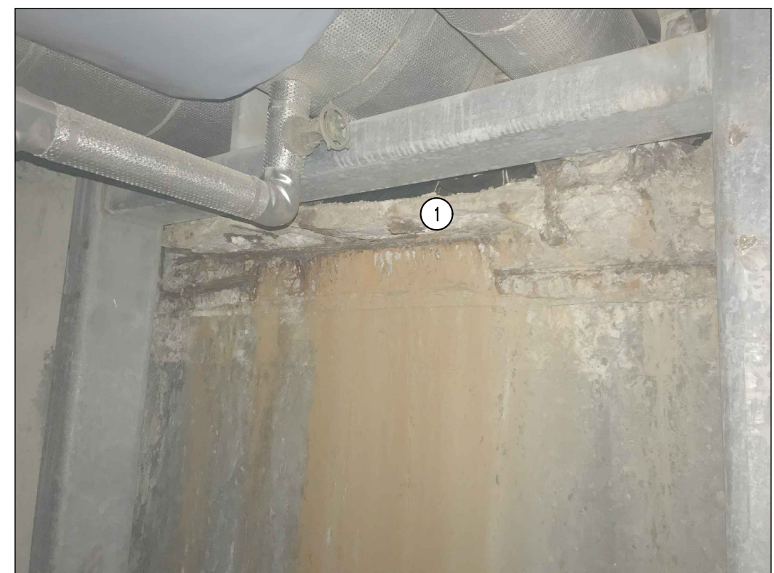
1 SPALLED CONCRETE, SEE REPAIR NOTE 1.
