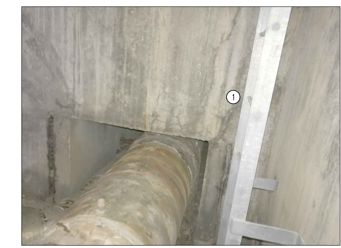
1 CONCRETE CRACK, SEE REPAIR NOTE 5.
