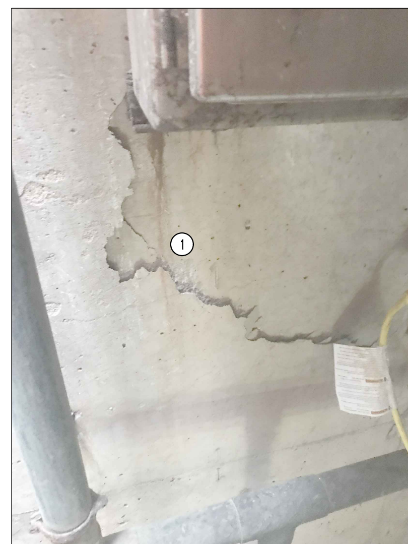
1 SPALLED CONCRETE, SEE REPAIR NOTE 3.
