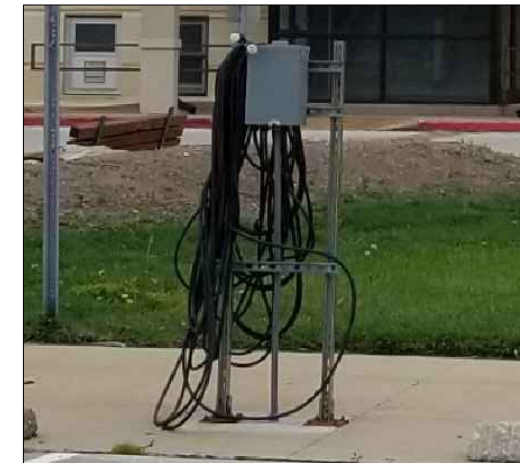
ITEM 24: AMBULANCE CHARGING STATION
